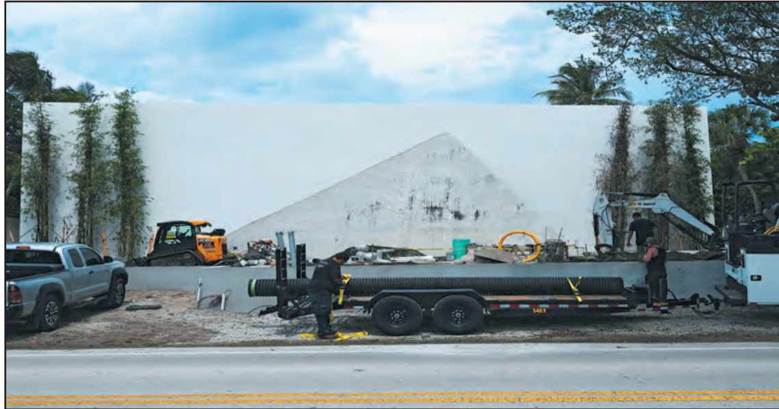
Workers deliver drainage pipe to the Ocean Boulevard property. The latest delay is an inability to get water and electricity without going under the road. Jerry Lower/The Coastal Star
