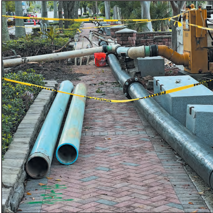
Repairs and cleanup are ongoing at the site of a sewer pipe that leaked into the Intracoastal Waterway near Marina Village. The breach in early July came in a section of pipe the city was seeking bids to replace. Tao Woolfe/The Coastal Star
