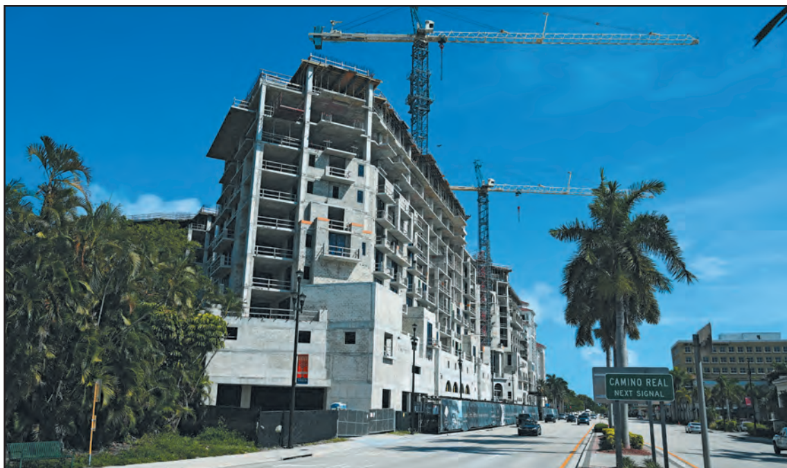
Cranes sat idle with few workers on site in July at the Mandarin Oriental, but in the city's overall view, 'they are actively doing work' on the project. Jerry Lower/The Coastal Star
