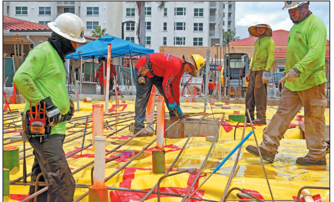
Employees from Proshell Construction Services Inc. install rebar while employees from Pomeroy Electric Incorporated install conduit during the construction of the new fire station on State Road A1A in front of Highland Beach Town Hall. Tim Stepien/The Coastal Star
