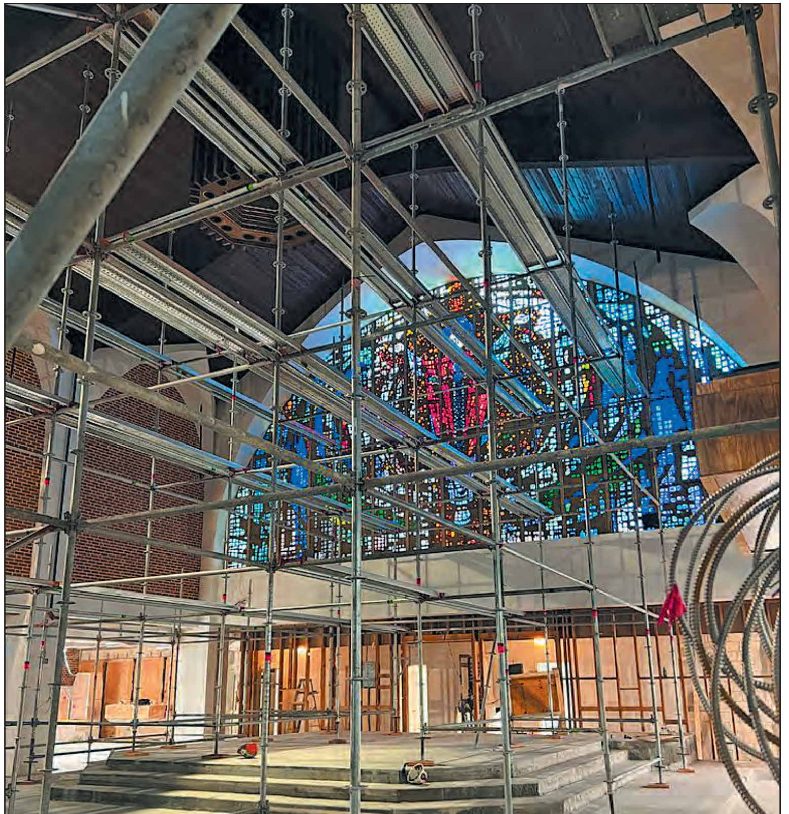
St. Gregory's Episcopal Church in Boca Raton began extensive remodeling in May. St. Gregory's leadership expects the work to finish by the end of November, just in time for the church's 70th anniversary. Photo provided
