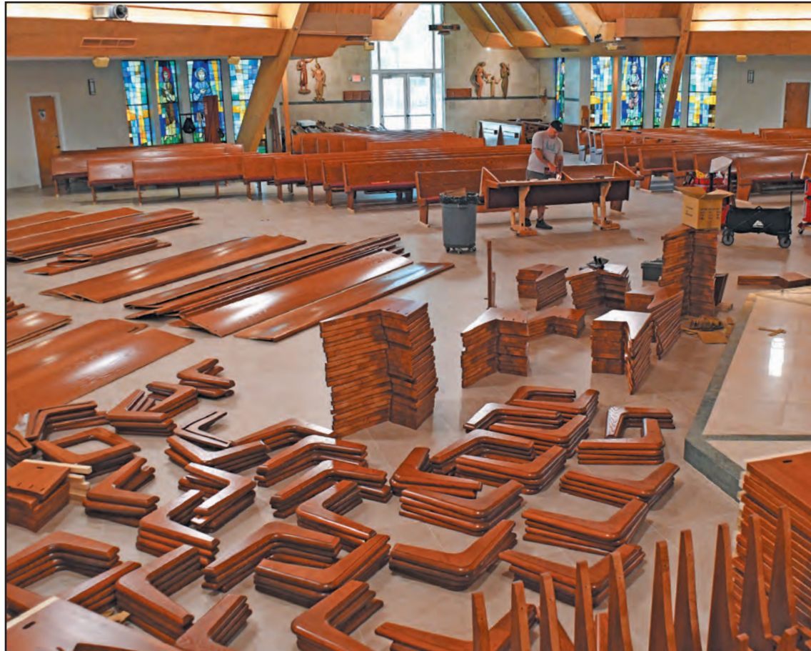
Contractor Coy Eaton assembles the new pews, which are a bit darker than the old ones, at St. Vincent Ferrer Catholic Church in Delray Beach. Jerry Lower/The Coastal Star
