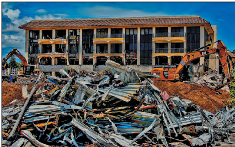
Former Atlantic Plaza buildings are being torn down to make way for the second phase of Atlantic Crossing. Tim Stepien/ The Coastal Star
