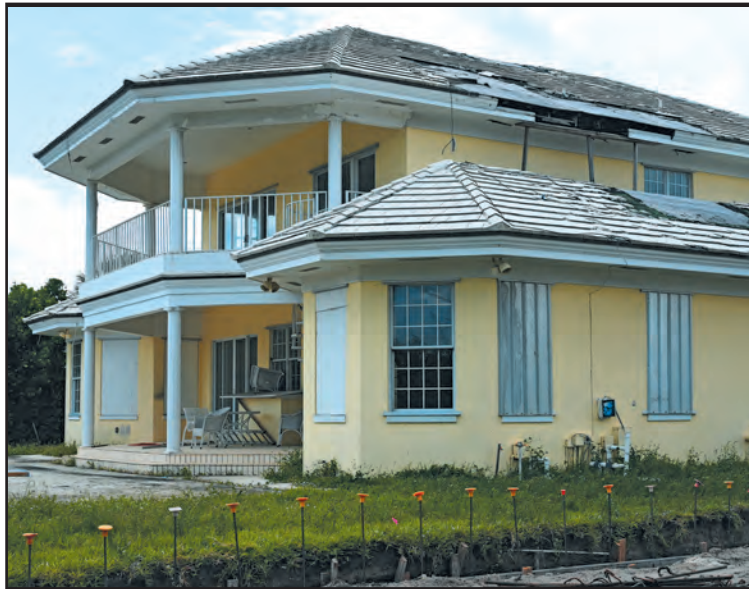
Temporary window coverings are just one of numerous problems for the house at 2900 Avenue Au Soleil, which the town hopes will be demolished. Jerry Lower/The Coastal Star
