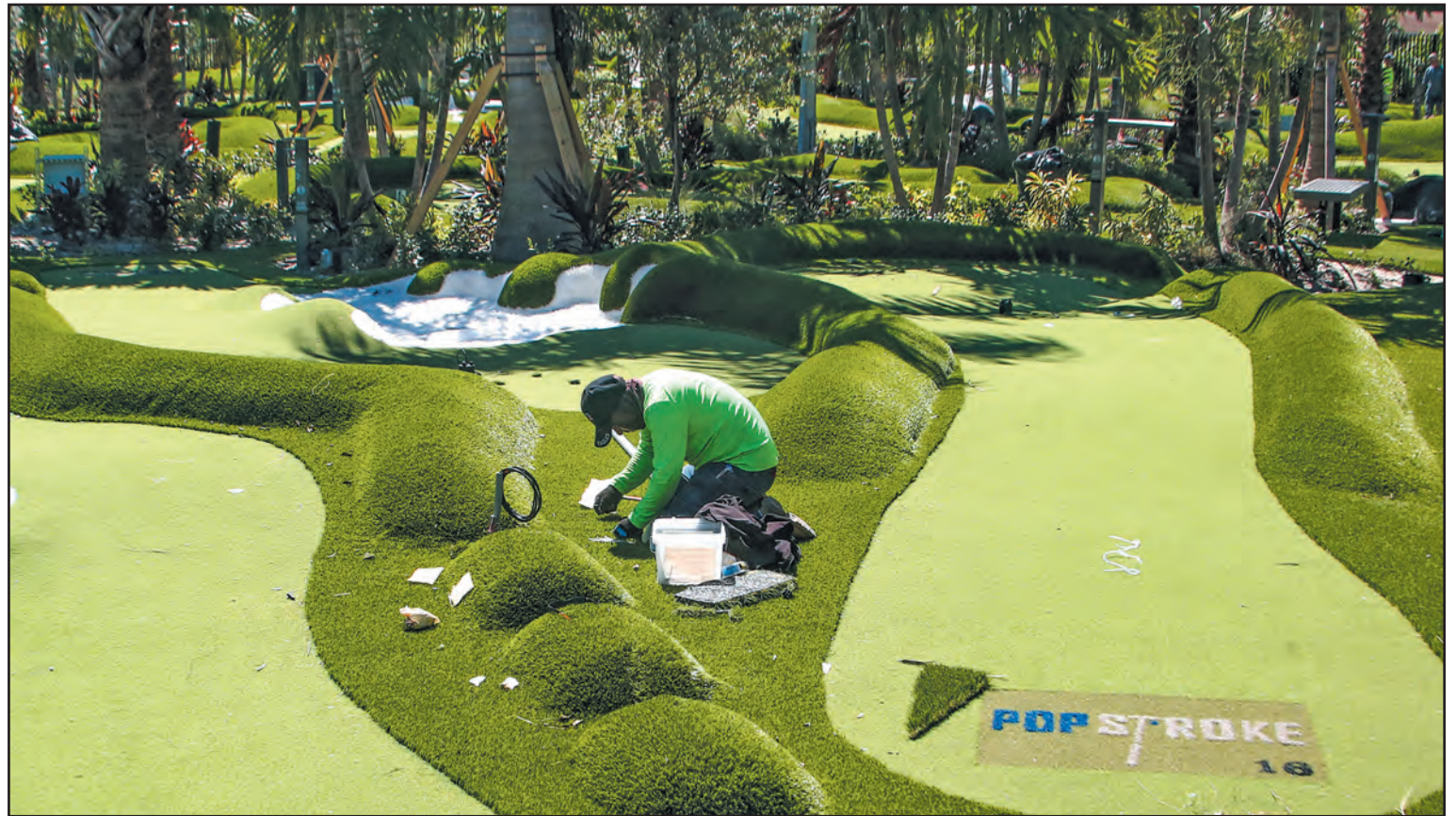
Construction of PopStroke in Delray Beach was in full swing in October. The 36-hole venue designed by Tiger Woods’ company is set to open the first week of November. Tim Stepien/The Coastal Star
