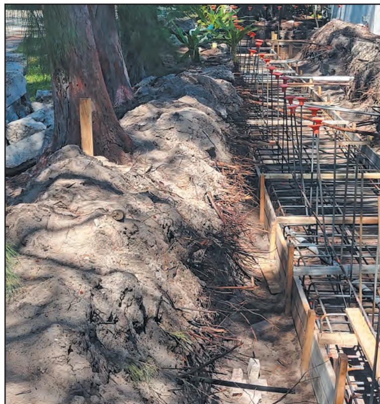
Work to replace a privacy wall came too close to more than a dozen Australian pines and their roots. Photo provided
