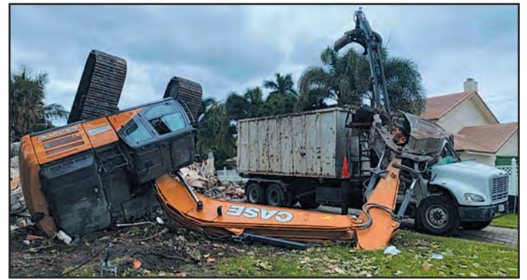
A construction worker died Nov. 9 when an excavator toppled over onto him at a home demolition in Delray Beach. Photo provided by Delray Beach Fire Rescue
