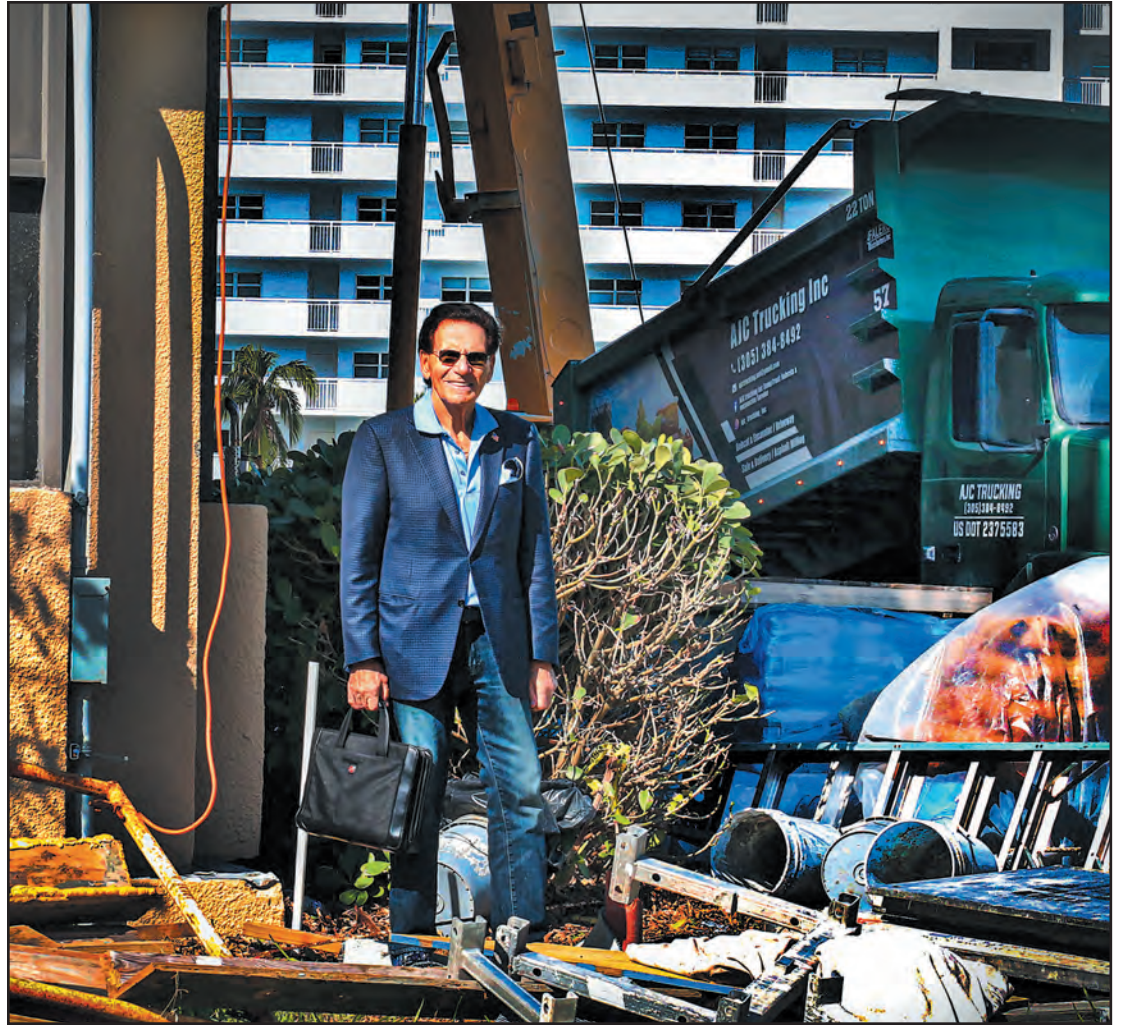
Jason Chudnofsky, board president of the Coronado, stands amid exterior repair work underway at the 336-unit Highland Beach condo. Tim Stepien/The Coastal Star
