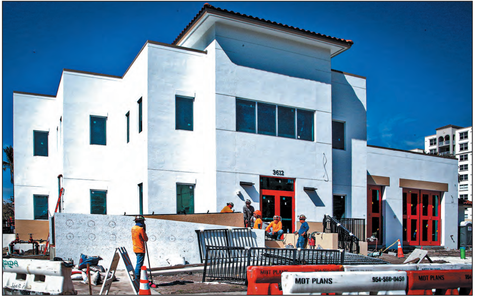
The new Highland Beach fire station in mid-February. It has a two-bay garage to house a ladder truck and a rescue vehicle. The old station will house a backup rescue vehicle and a backup fire truck. Tim Stepien/The Coastal Star
