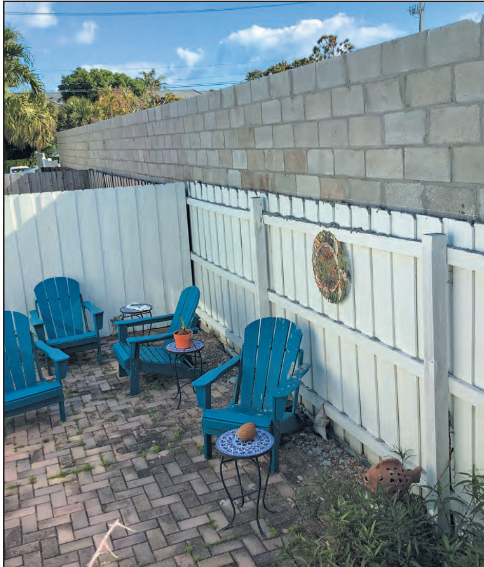
A newly built concrete block retaining wall at Siréne Villas overshadows a neighbor's existing wooden privacy fence. Photo provided
