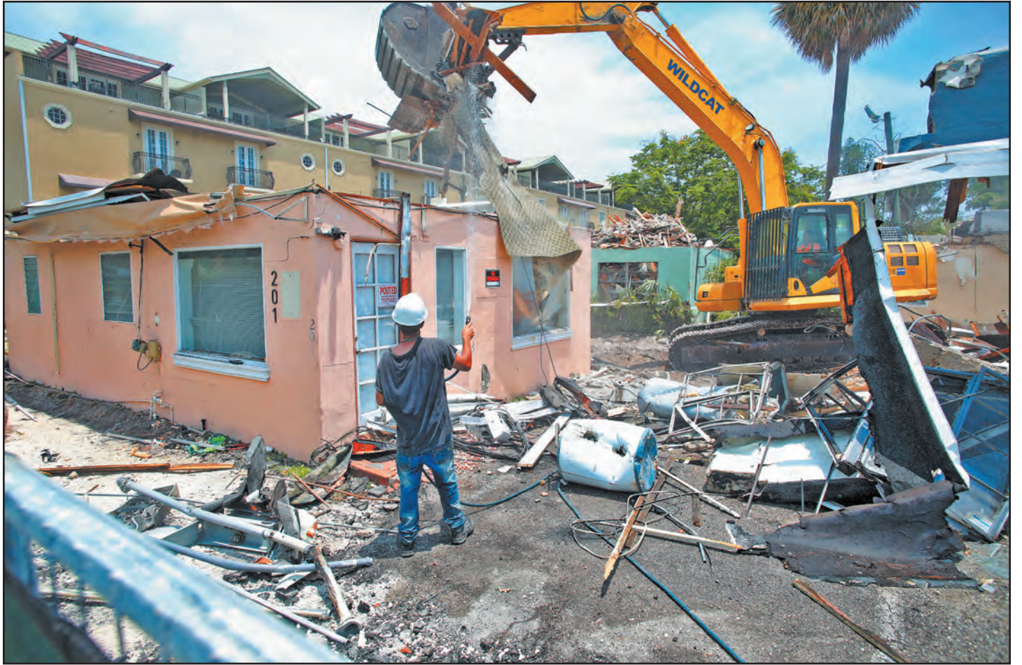
Demolition of Key West-style cottages on the north side of Ocean Avenue began in mid-May. Mayor Karen Lythgoe is optimistic that a developer will negotiate a long-term lease with the property owners. Tim Stepien/The Coastal Star
