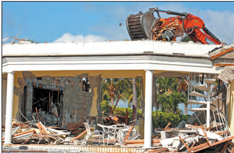
Demolition equipment tears apart the home at 2900 Avenue Au Soleil in mid-May. Tim Stepien/The Coastal Star
