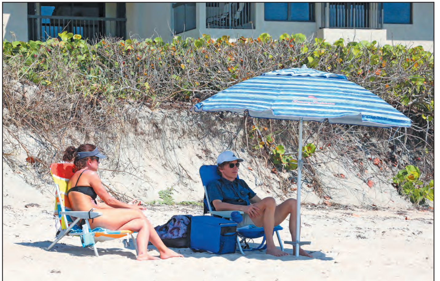
Natalie Gauthier and Michael Crouteau from Quebec lounge by a cliff of sand in May just north of Boynton Beach Oceanfront Park. The erosion and dead vegetation reflect past storm damage. Tim Stepien/The Coastal Star
