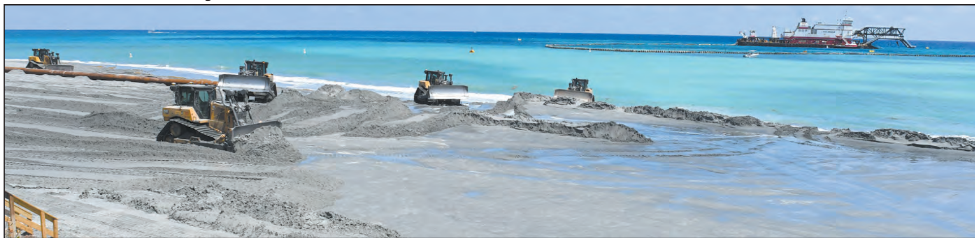
Five bulldozers level freshly pumped sand after it was spread onto the beach in Ocean Ridge from the dredge (at right) as part of a $9.4 million U.S. Army Corps of Engineers project. The gray color comes from organic sediment and is common for beach renourishment projects. It will change over time to the natural color of sand. The project is expected to continue through April, before the peak of sea turtle nesting season arrives. Jerry Lower/The Coastal Star
