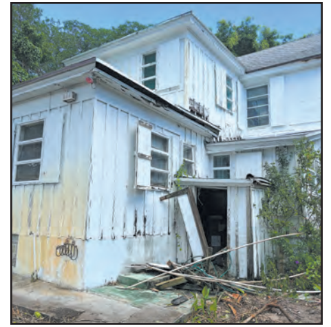
One source of cats was this building, which had been covered in brush. The owners plan to build a new home. Jerry Lower/The Coastal Star
