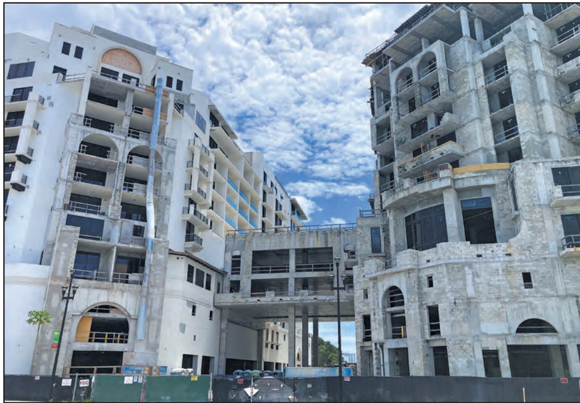
Construction work is still not completed at the Mandarin Oriental. The condo residences, with plastering, are to the left and the hotel is to the right. Larry Barszewski/The Coastal Star
