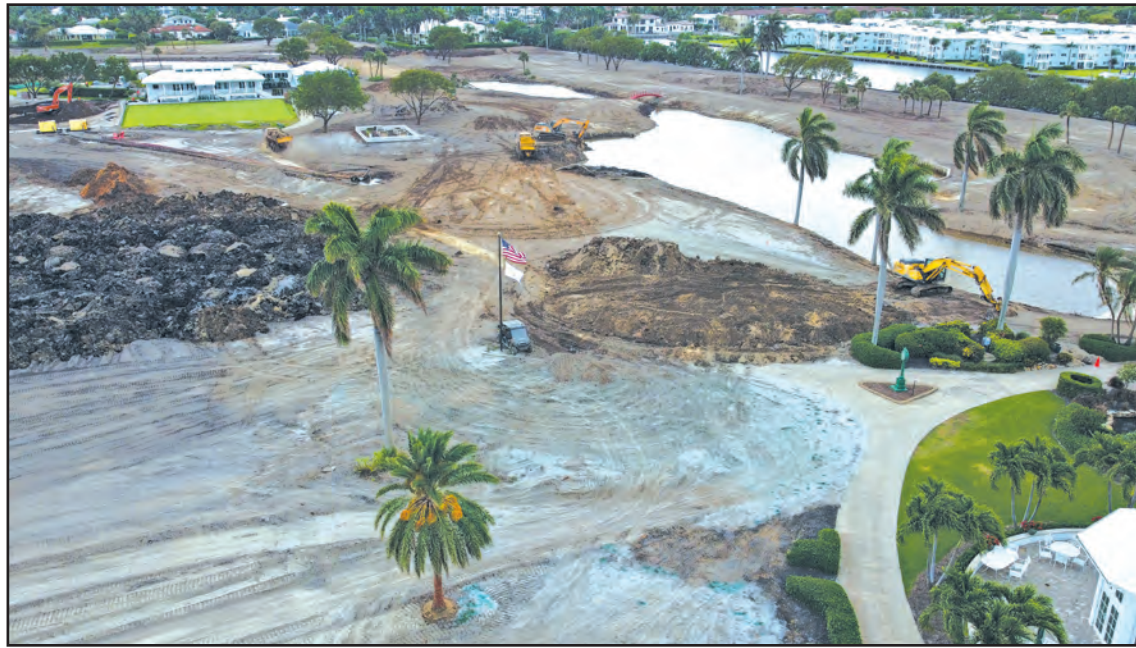
Bulldozers and backhoes work the grounds of The Little Club as part of the remake of the property. Jerry Lower/The Coastal Star
