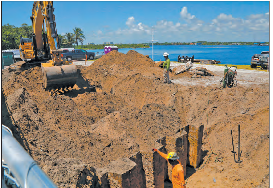
Earth-moving equipment and workers are busy at 1960 S. Ocean Blvd. in Manalapan on June 29. The work is taking place on David MacNeil's side of the property that he and fellow multibillionaire Larry Ellison agreed to split. Combined, the two men have invested hundreds of millions of dollars in Manalapan real estate recently. Tim Stepien/The Coastal Star
