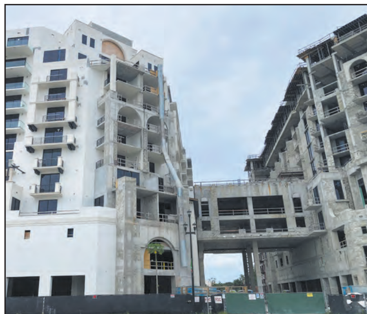
Construction work remains incomplete at the Mandarin Oriental. The condos, with plastering, are to the left and the hotel is to the right. Larry Barszewski/The Coastal Star
