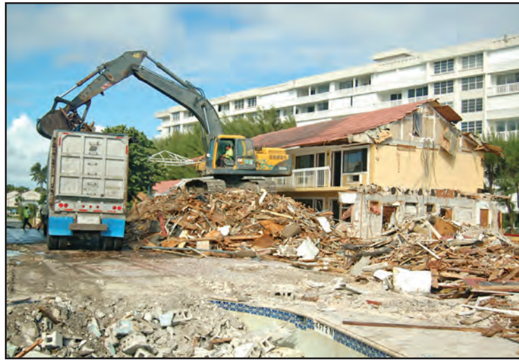
The developer has begun a limited demolition of the Oceanfront Inn in South Palm Beach. Willie Howard/The Coastal Star
